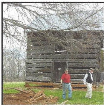
The barn is leaning and needs to be stabilized.
